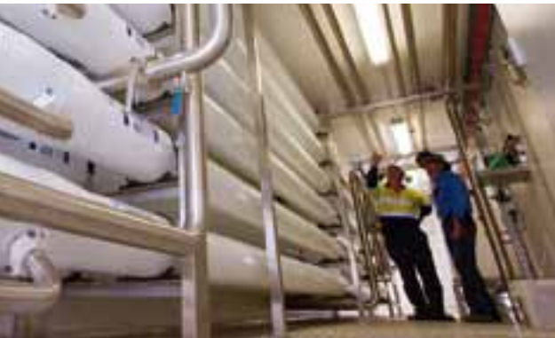
Santos employees inspect a reverse osmosis water treatment facility at the Fairview plantation, eastern Queensland.
