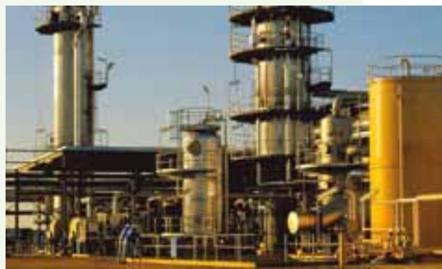
Ballera gas plant CO 2 train.
