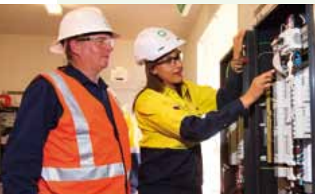
Control system hardware.
